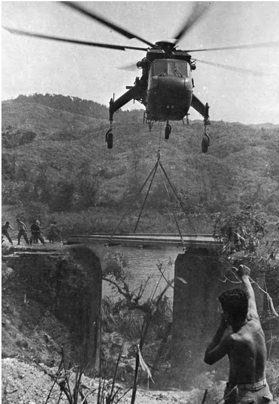
An Army CH-54 Flying Crane lowers a dry span bridge over a gap as the Marine 11th Engineer Battalion worked to reopen Highway 9 to Khe Sanh during Operation PEGASUS.
